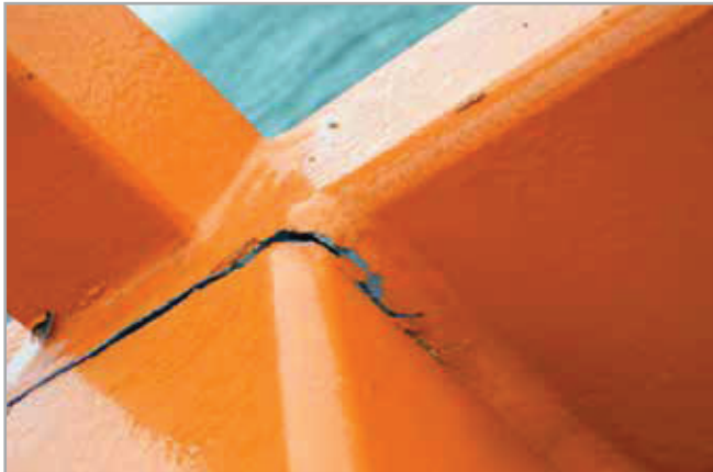
Typical crack due to fatigue damage.
